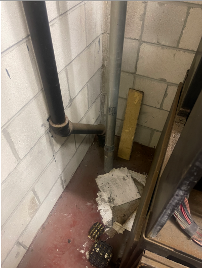
#15 machine room clean up needed
