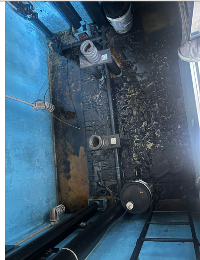
#16 Oil and water in pit
