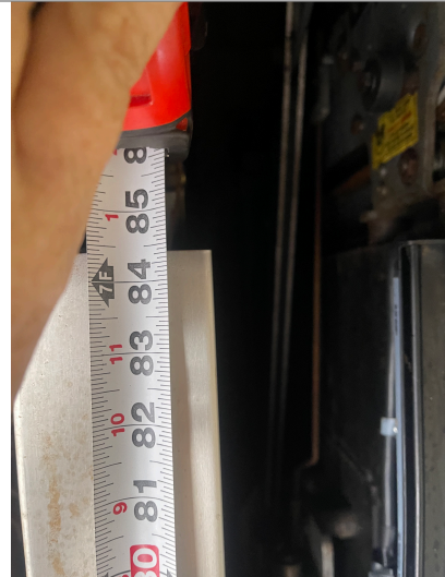
#28 door gap exceeds .5"
